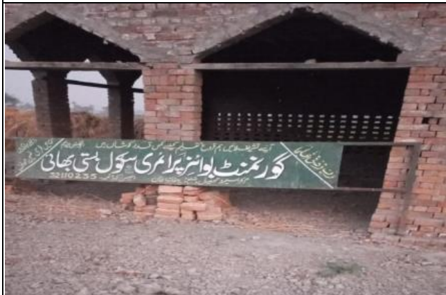
A view of under construction school building of GPS Basti Bhai Tehsil & District D.G Khan.
