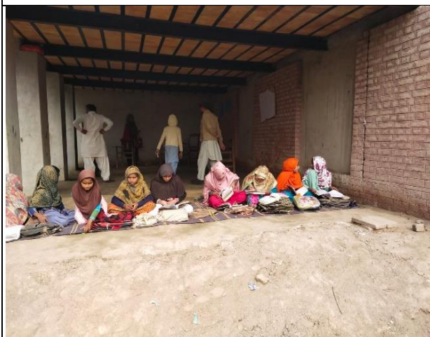
A view of Repairing Required at GPS Ghulam Mustafa Lolai Tehsil Khanpur, District Rahim Yar Khan
