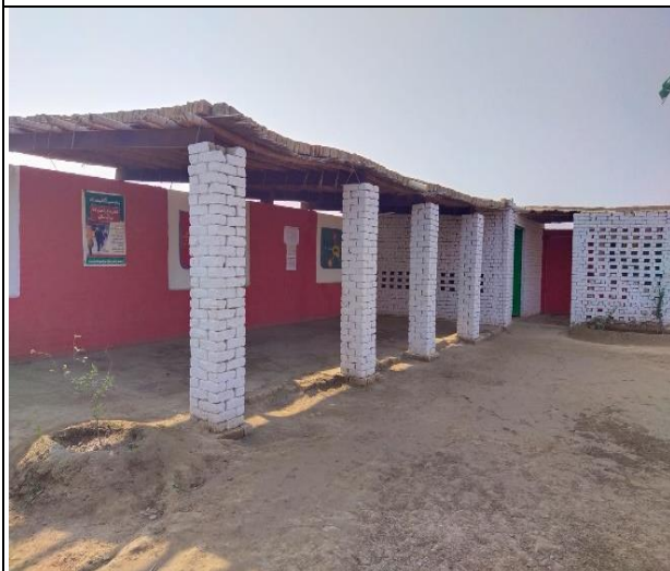
A view of Repairing Required at GPS Sheikh Jivenda Tehsil Taunsa, District D.G Khan
