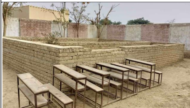
A view of Repairing Required at GPS Sadiq Abad Tehsil Jampur, District Rajanpur
