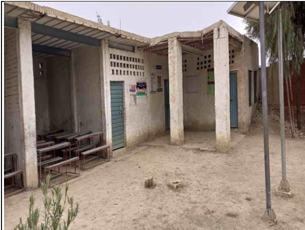
A view of Repairing Required at GPS Chak Chhina Tehsil Jampur, District Rajanpur.
